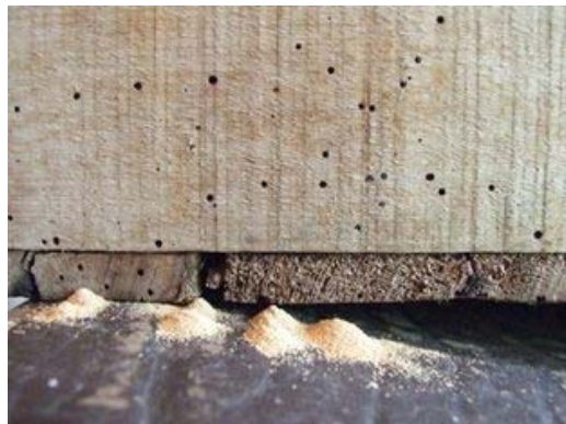
Anobium damage to timber - it can be several years before there are any outward signs of activity
